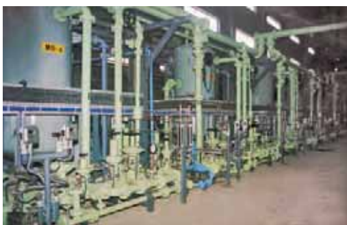
Annual maintenance of PLC based demineralisation plant at thermal power station
