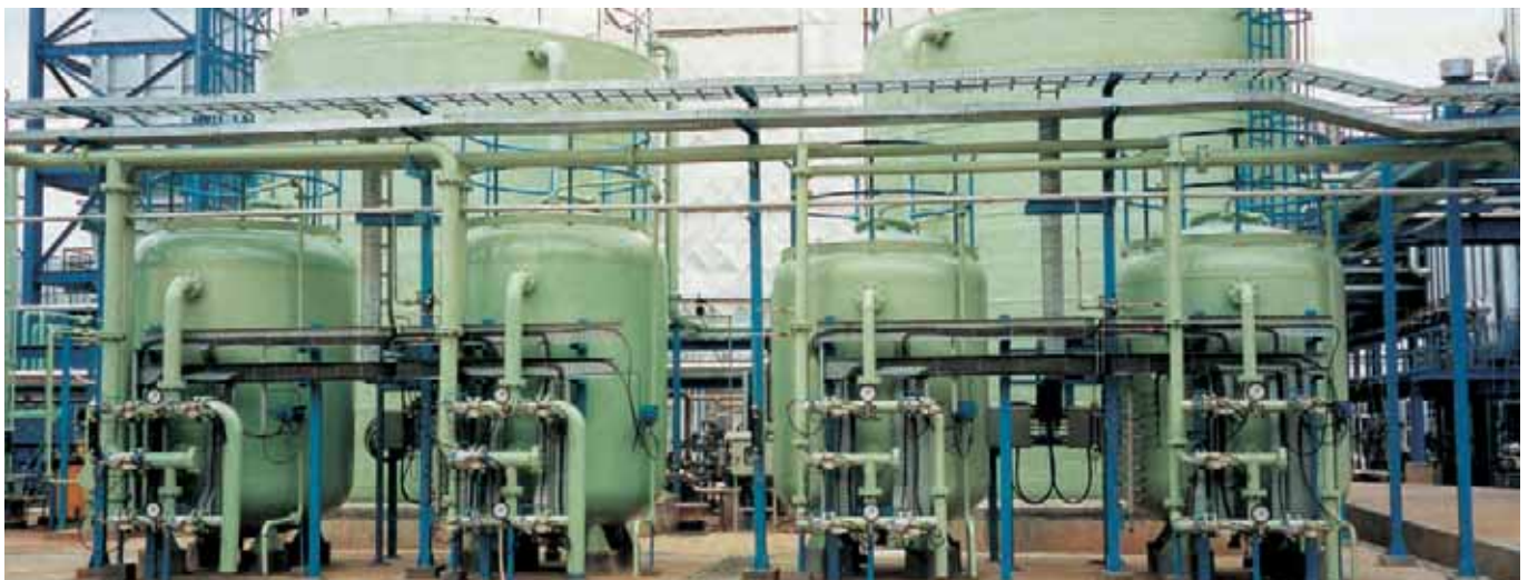
PLC based automatic demineralisation plant for thermal power station
