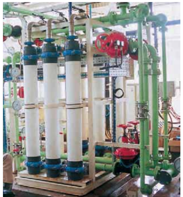
Ultra filtration system for raw water treatment
