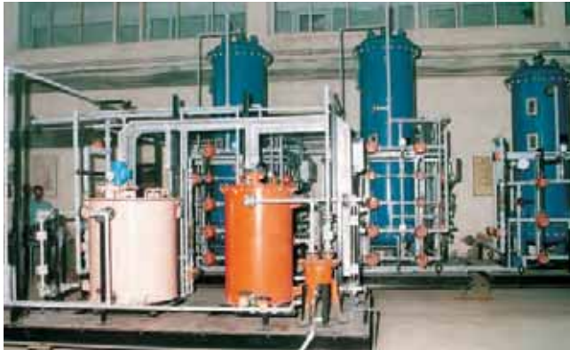
Brine softening plant for chlor alkali production
