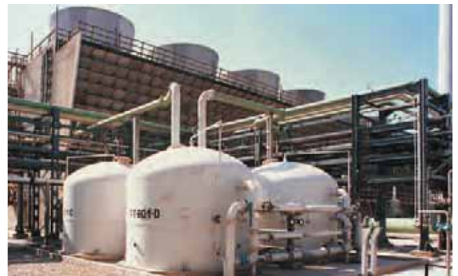
Cooling water treatment
