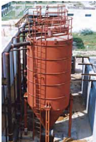
Continuous sand filters
