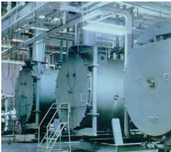
Boiler water treatment
