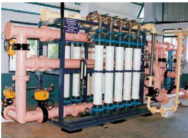
Plating effluent recycle plant at auto ancillary unit
