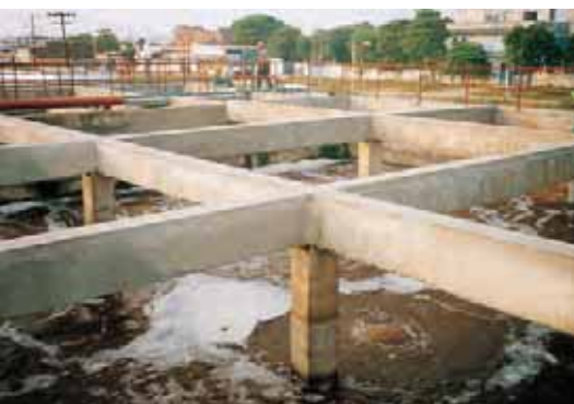
Sequential batch reactor for municipal sewage treatment
