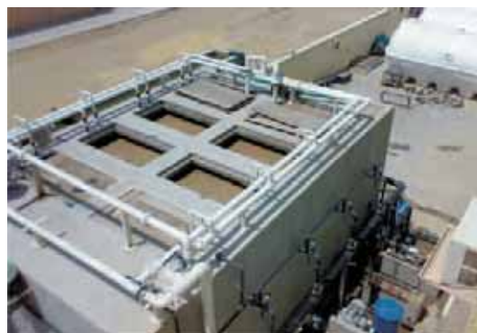
Membrane-bio reactor for sewage treatment at a civil contracting company
