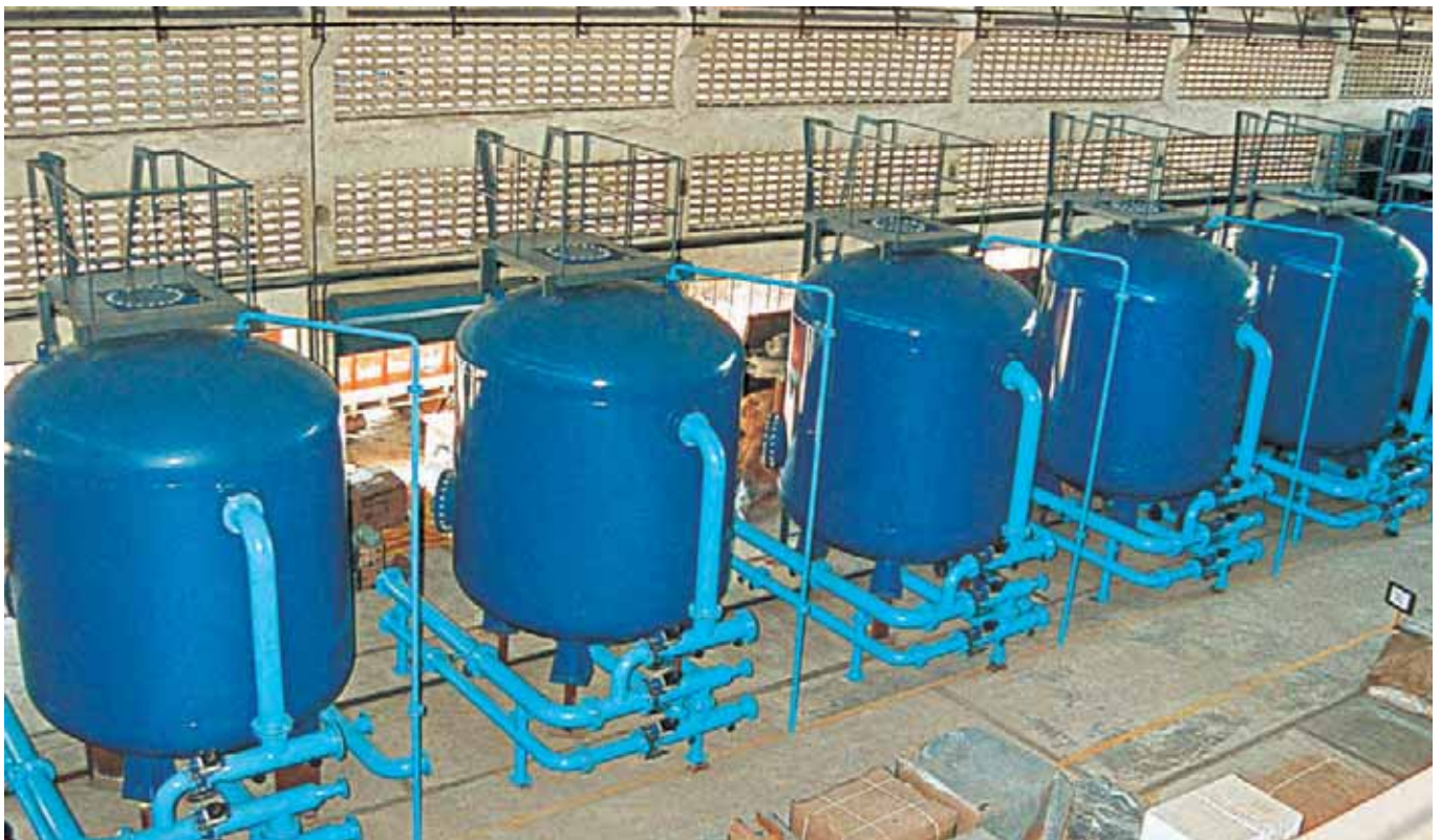
Pressure sand filters for city water supply
