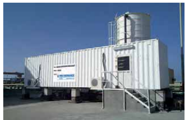
Brackish water treatment RO plant
