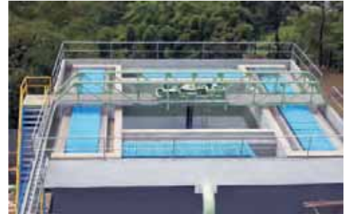
Ultra high rate clarifier
