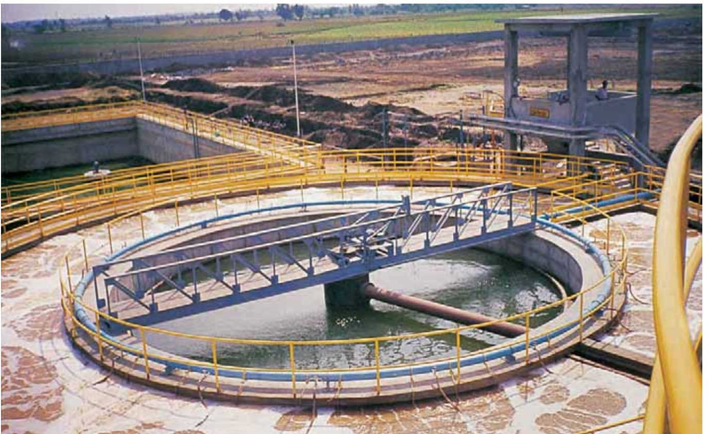
Textile waste water treatment plant
