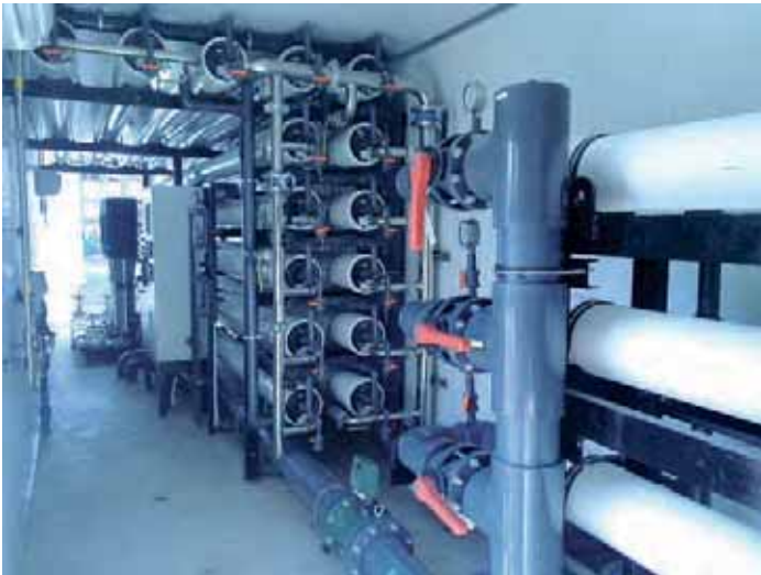
Containerised reverse osmosis plant
