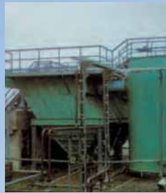
Inclined plate clarifier
