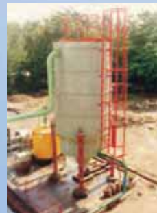
Continuous sand filter
