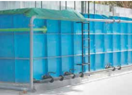
Fluidised media reactor for sewage treatment
