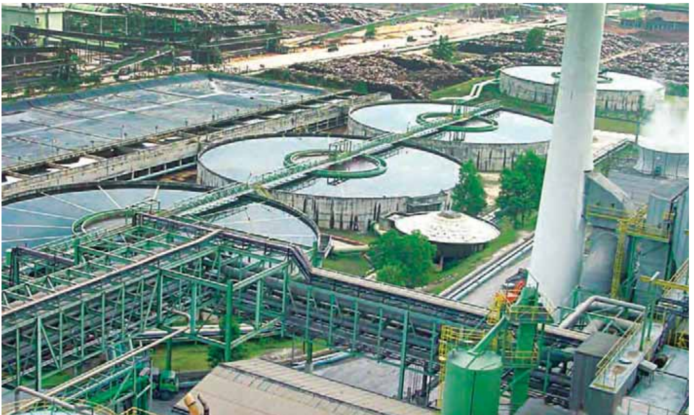
Aerial view of high rate solids contact clarifiers for pulp & paper mill
