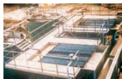
Inclined plate clarifier
