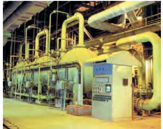
Condensate polishing units for thermal power station
