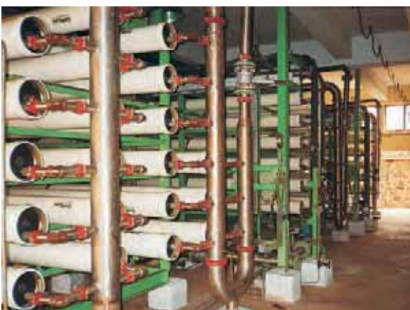
Membrane based zero discharge plant at petrochemical complex
