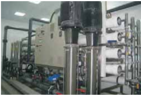
Reverse osmosis plant for packaged drinking water
