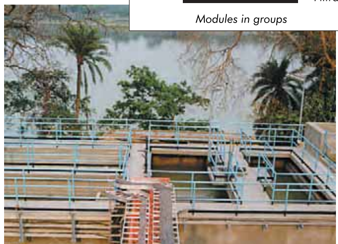
Submerged membrane bio-reactor for recycle of industrial and municipal effluent
